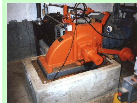
Fig. 3: Turbine with generator
