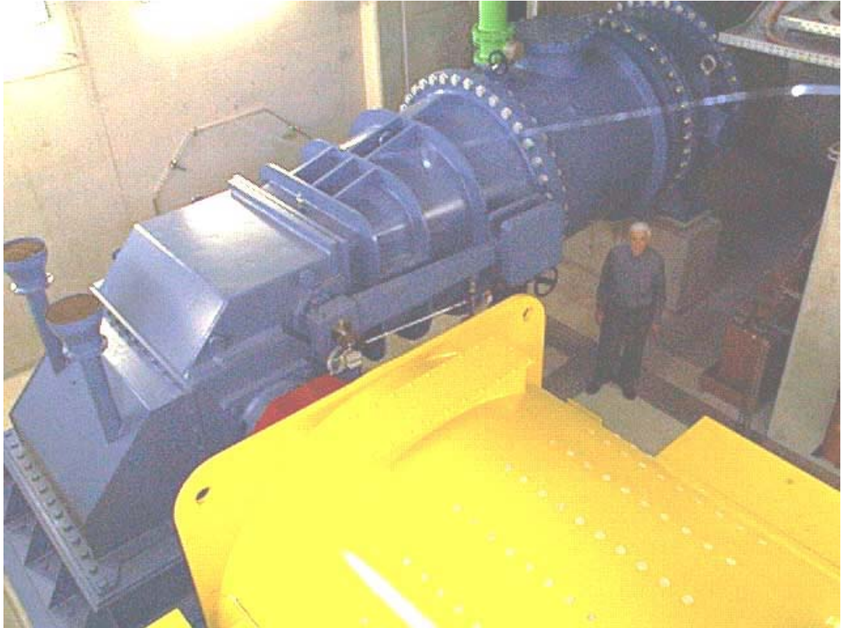
Fig. 6: Power train in the power house
